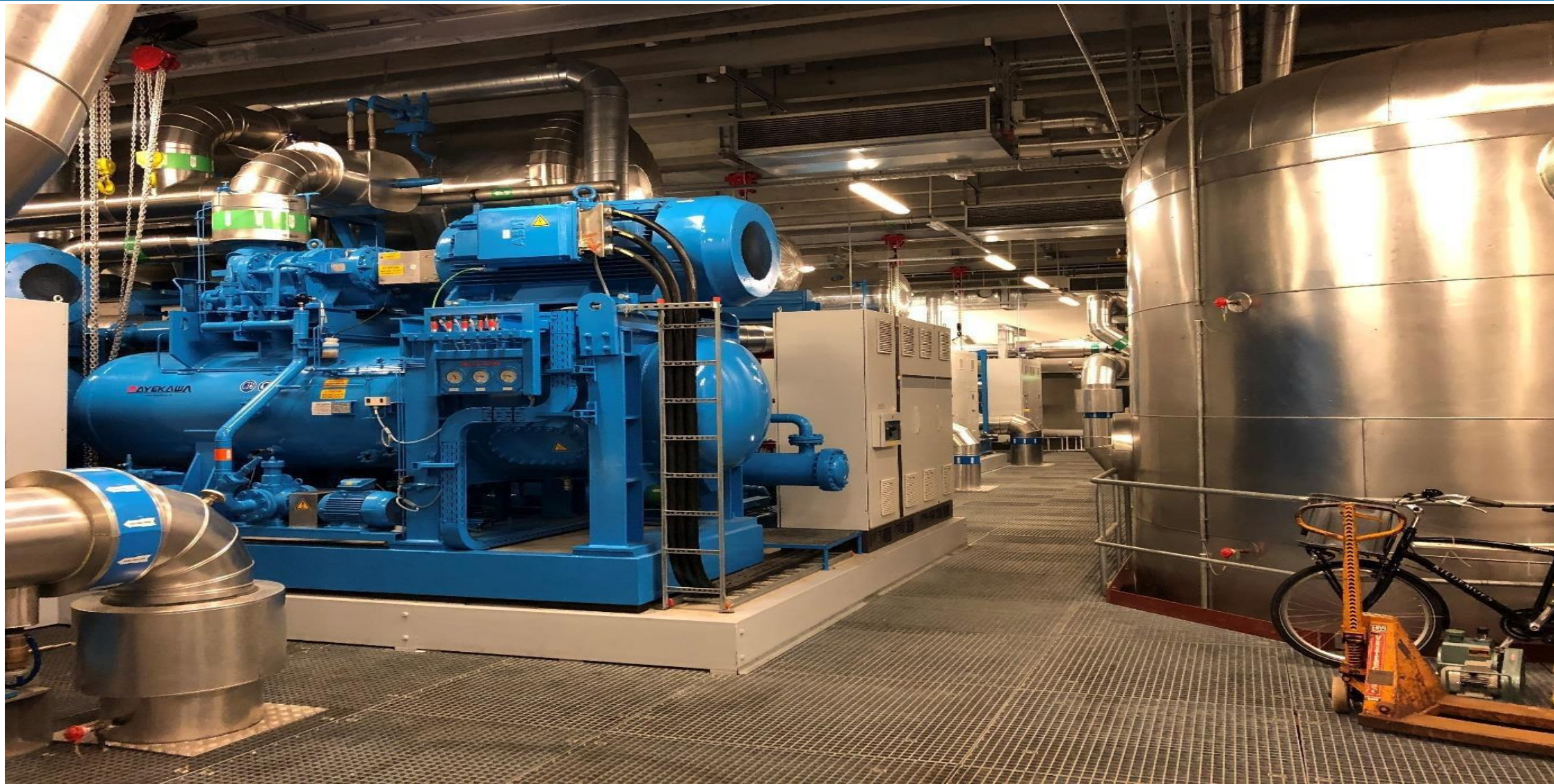
HOFOR's DC Plant in Adelgade Copenhagen
